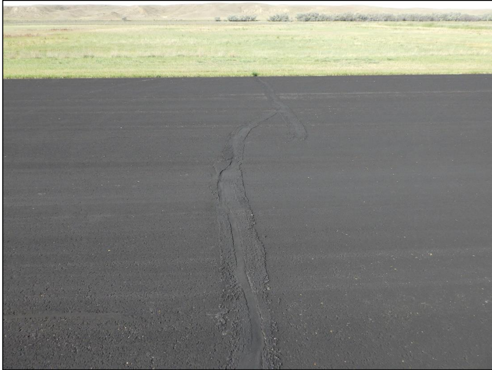
RW08-01-47: L&T Cracking
