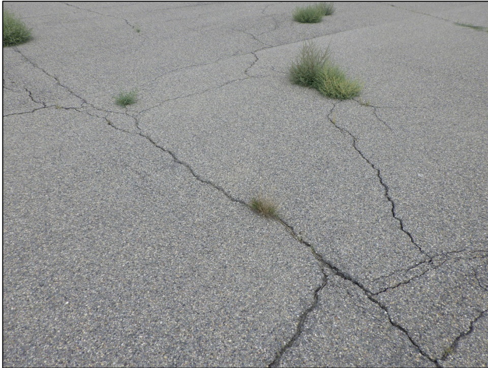
AP01-02: Block Cracking
