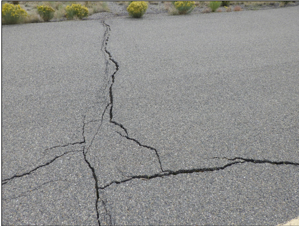
TW01-01: L&T Cracking
