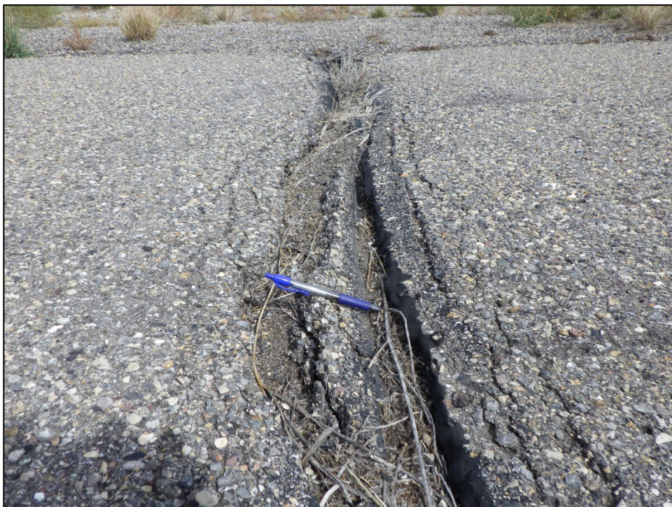
RW14-02-16: L&T Cracking
