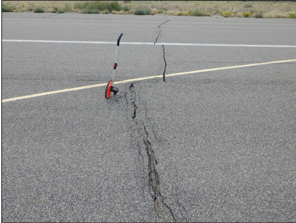
RW14-01-55: L&T Cracking
