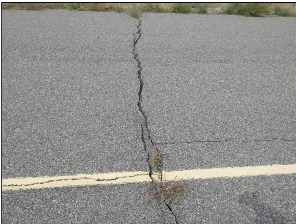
TW01-02: L&T Cracking
