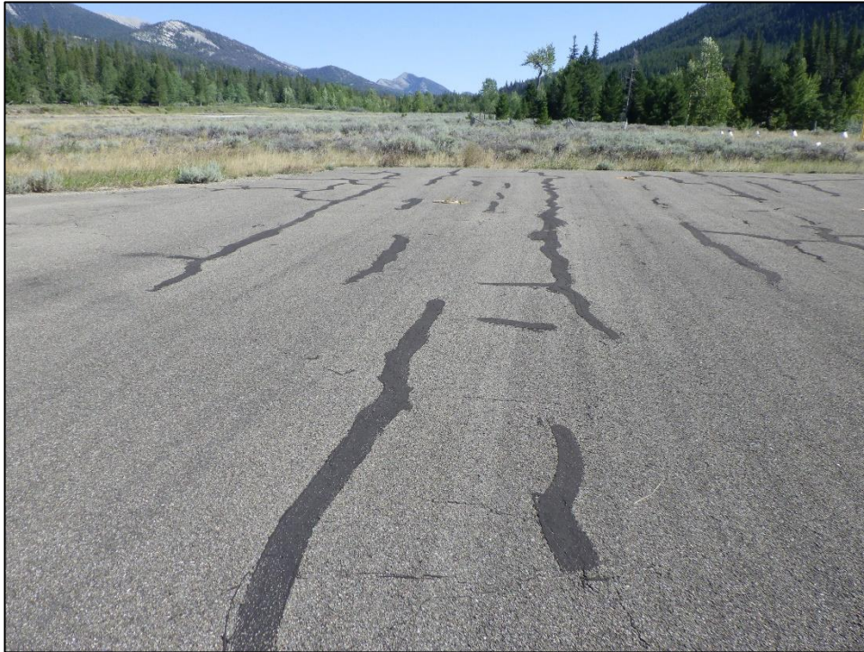
AP01-05: L&T Cracking
