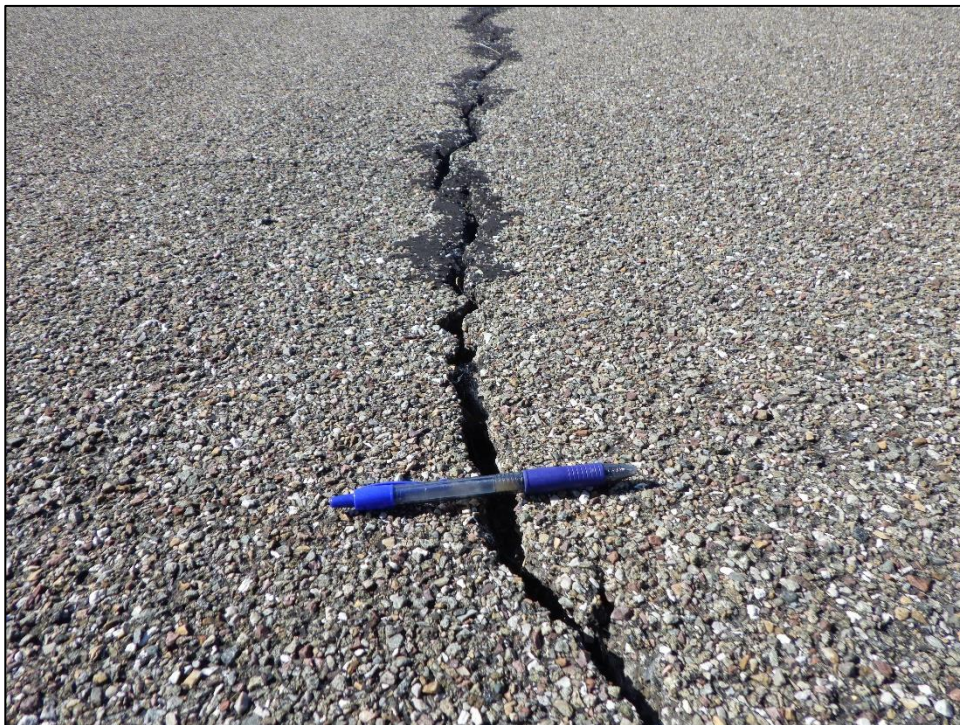
AP01-05: L&T Cracking
