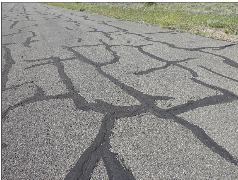
RW12-01-66: Block Cracking
