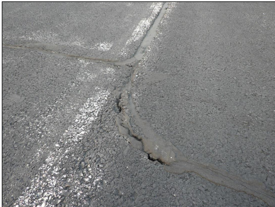
RW04-02-44: L&T Cracking
