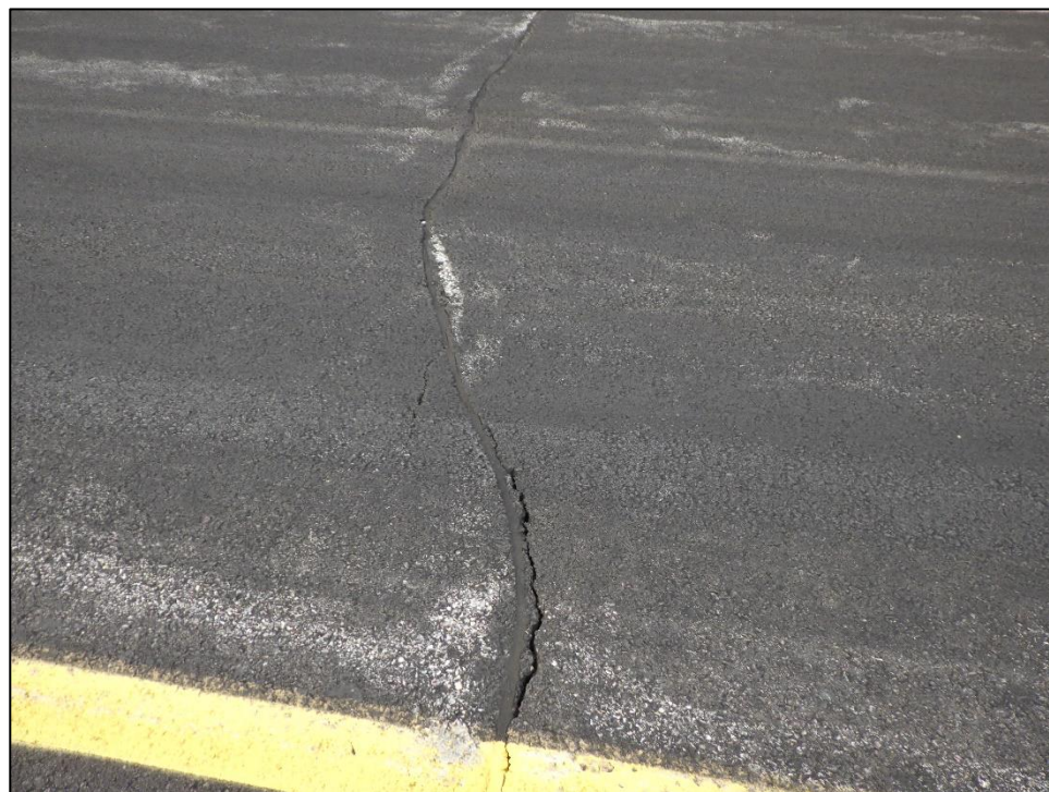
TW04-01: L&T Cracking
