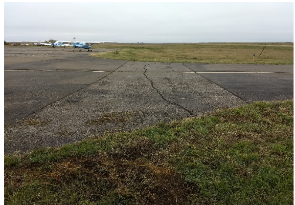
T-2, Patch and Crack
