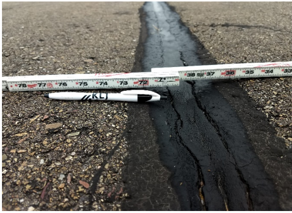
R-1, Crack and Depression
