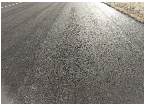
R-1, Overview with Bleeding
