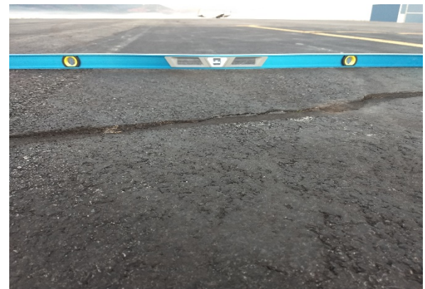
A-2, Depression and Cracking
