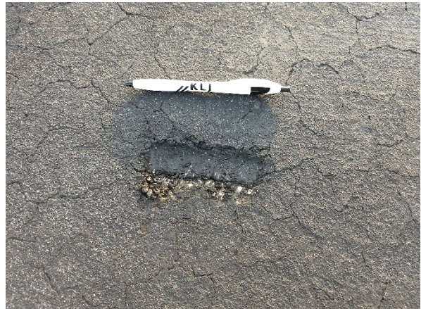
A-1, Raveling and Depression
