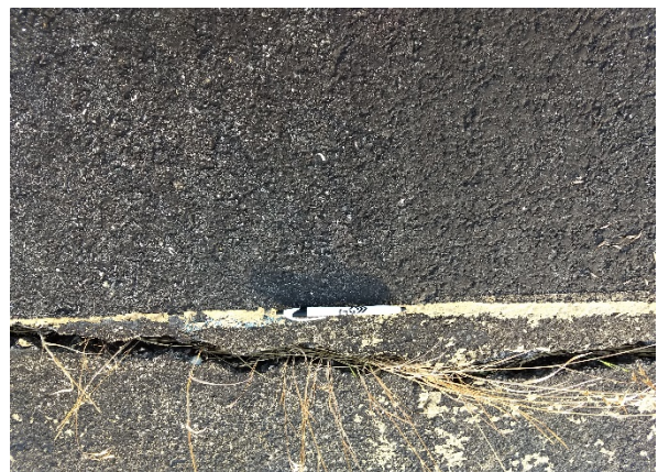
T-4, Crack with Vegetation
