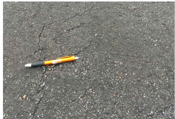
R-11, Slip Crack
