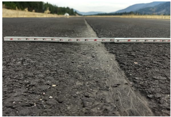
T-11, Depression and Sealed Crack
