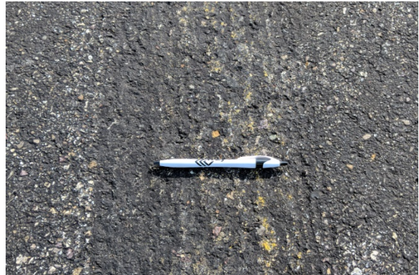
T-11, Raveling - Paint Grind
