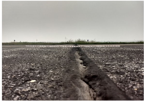
T-3, Depression and Crack with Failed Sealant
