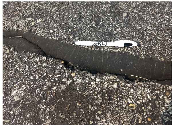
A-2, Crack with Failed Seal
