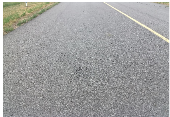
T-4, Bleeding and Crack
