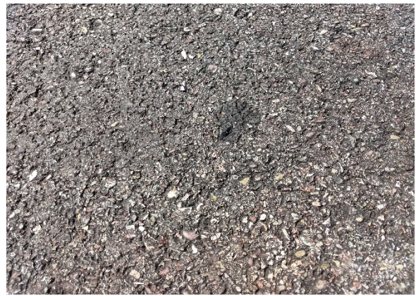
T-11, Surface Detail and Spilled Oil
