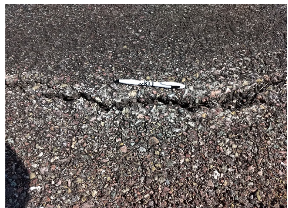
R-11, Crack and Mechanical Raveling
