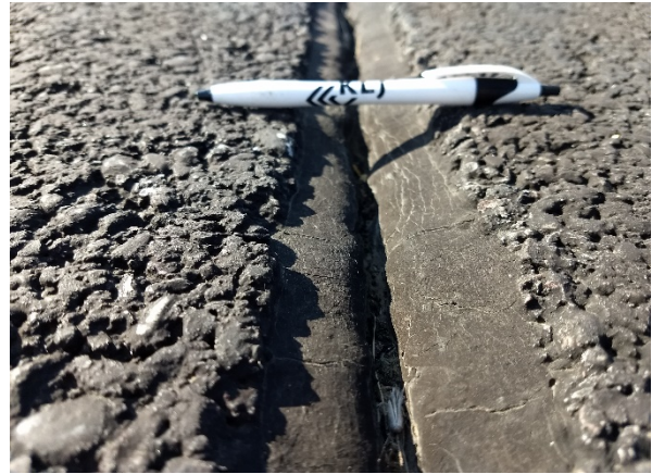
A-1, Crack and Depression
