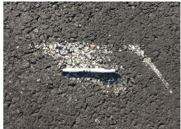
R-1, Mechanical Raveling
