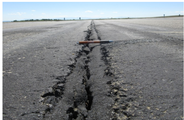
R-4, Cracking-Failed Sealant
