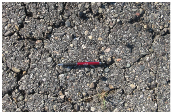
T-1, Alligator Cracking
