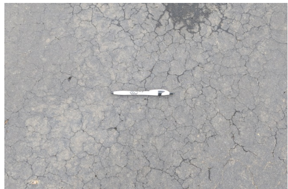
A-11, Dense Grade - Raveling
