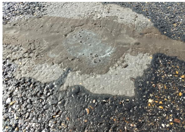
R-22, Sealed Crack and Patch
