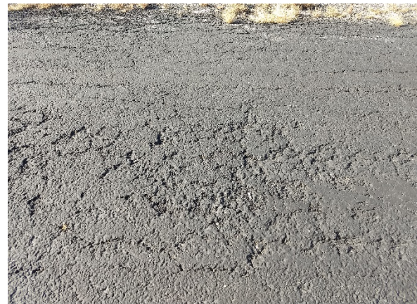
T-2, Surface with Raveling
