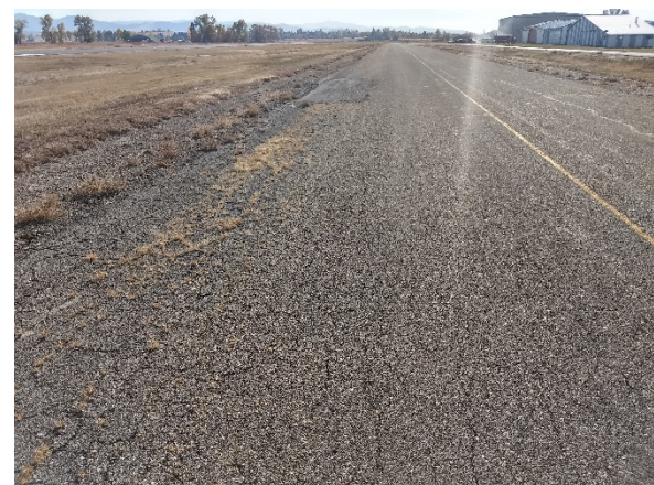
T-3, Alligator Cracking and Patch
