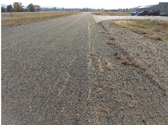
T-3, Overview with Alligator Cracking
