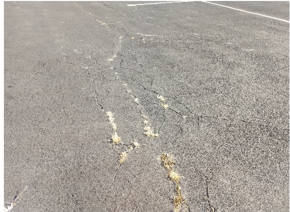
A-1, Alligator Cracking
