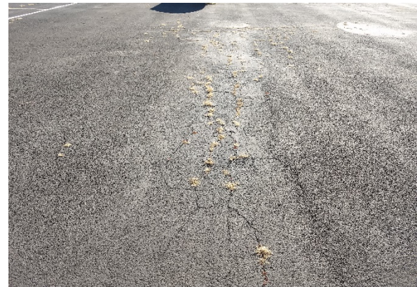
A-2, Alligator Cracking and Depression
