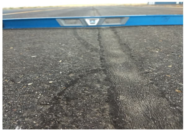
T-2, Sealed Crack with Depression
