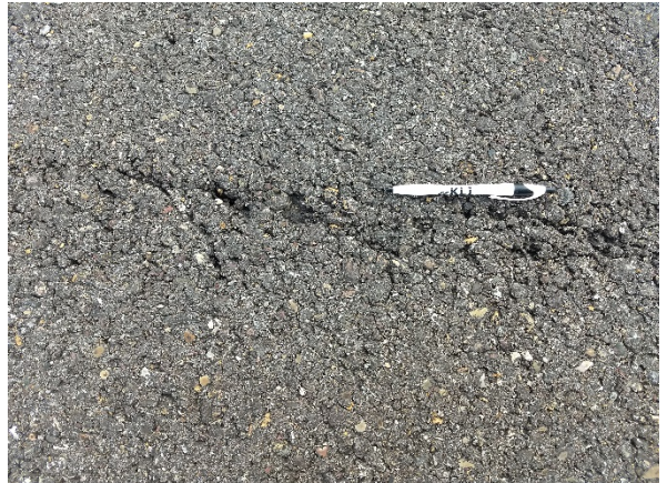
R-1, Mechanical Raveling
