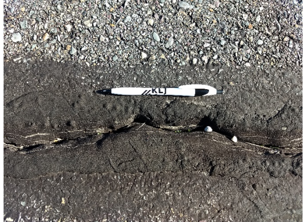
A-1, Crack with Failed Sealant
