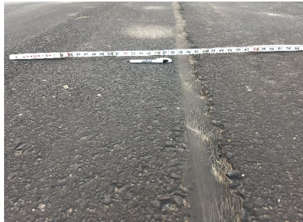
A-1, Crack and Depression
