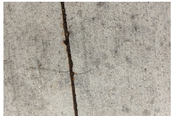
A-2, Joint Spall and Crack
