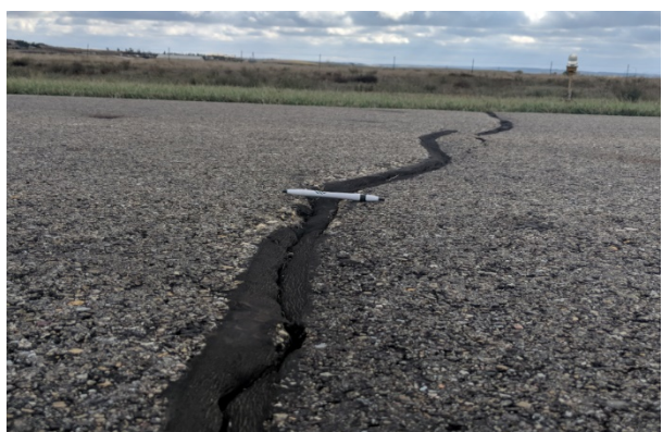
R-1, Crack Depression
