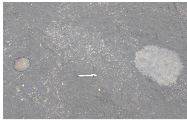
A-2, Fuel Spill Patch
