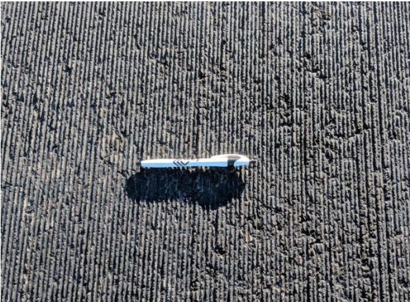
A-1, Raveling, Surface Grind
