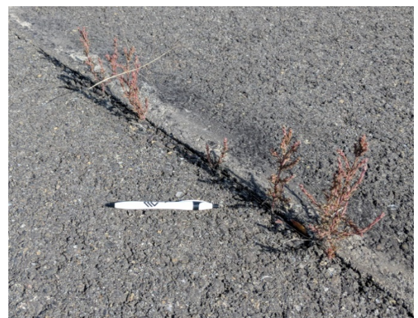
T-3, Crack Vegetation
