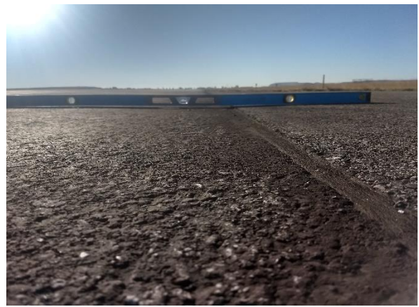
R-2, Crack with Depression
