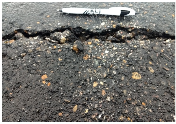
T-1, Crack with FOD
