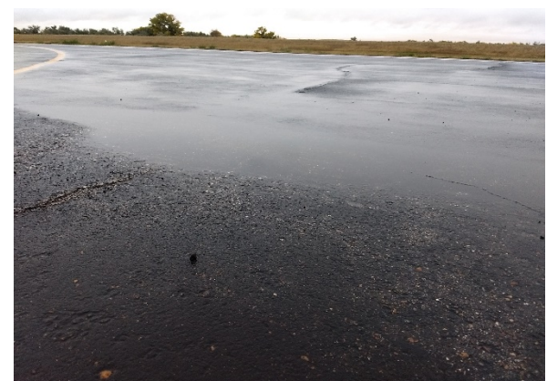
R-1, Depression with Crack
