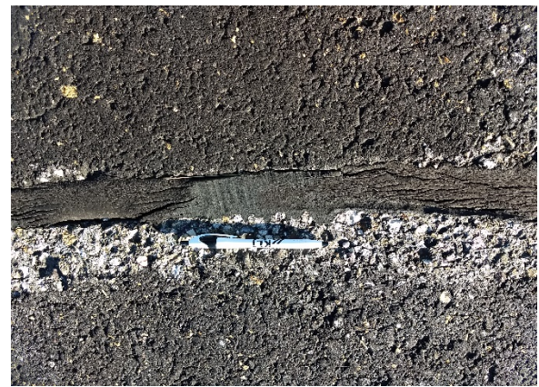
T-13, Sealed Crack with Mechanical Raveling
