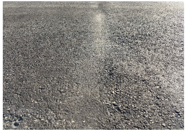
T-2, Depression with Pooled Surface Sealant
