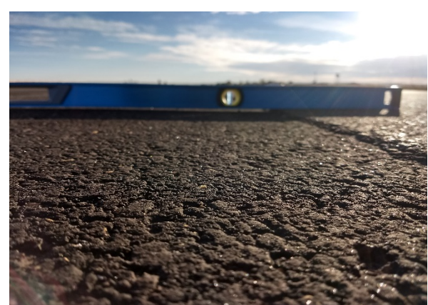
R-13, Depression along Joint
