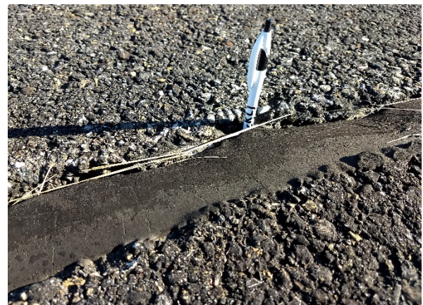
A-11, Crack with Failed Sealant
