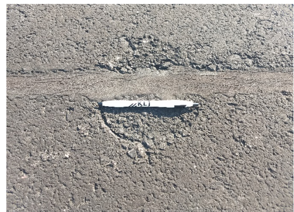
R-1, Patch with Crack
