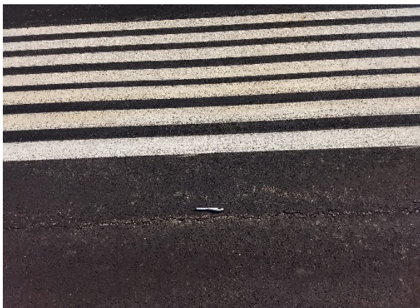
R-1, Overview with Crack
