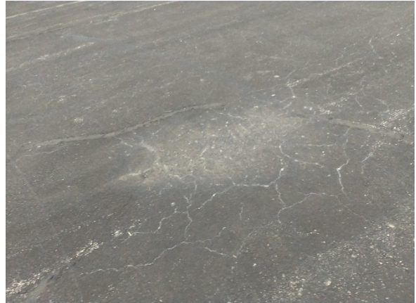
T-4, Depression with Cracks
