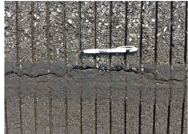
R-1, Grooved Surface and Crack
