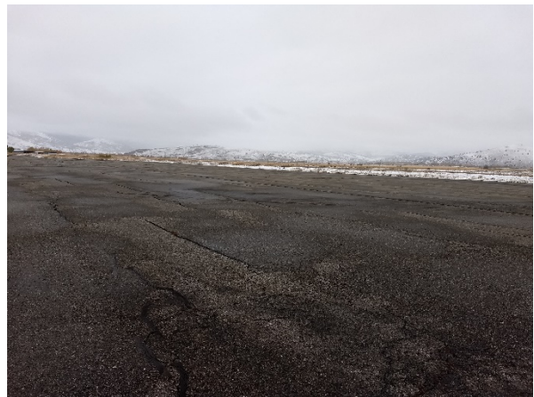
A-1, Surface Weathering with Cracks
