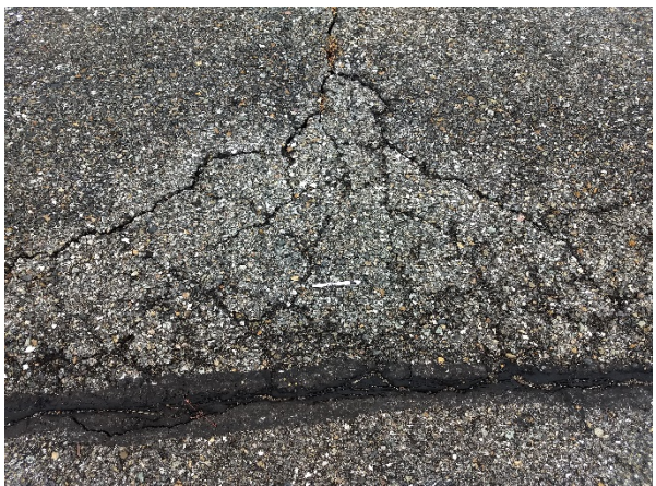
A-2, Crack with Depression
