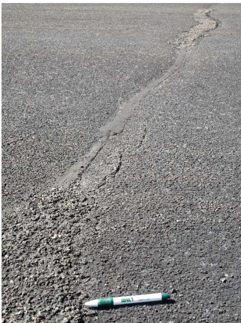
T-1, Surface detail with cracking and patch
