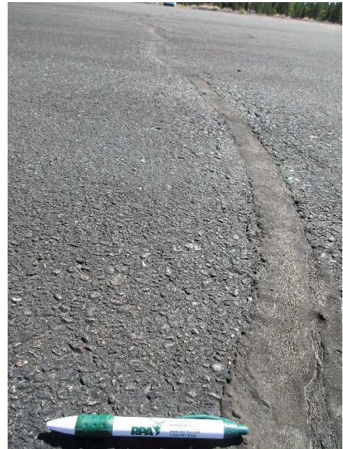
A-4, Surface detail with cracking
