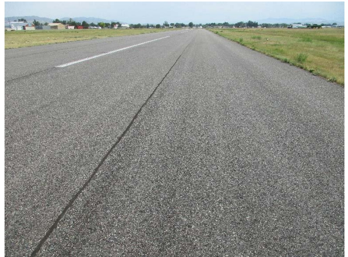
R-1 , Overview with cracks
