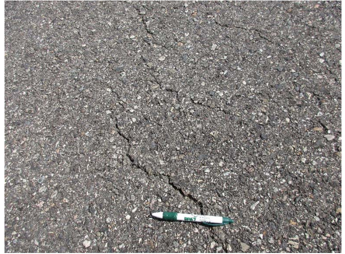
A-1 , Surface detail with cracking
