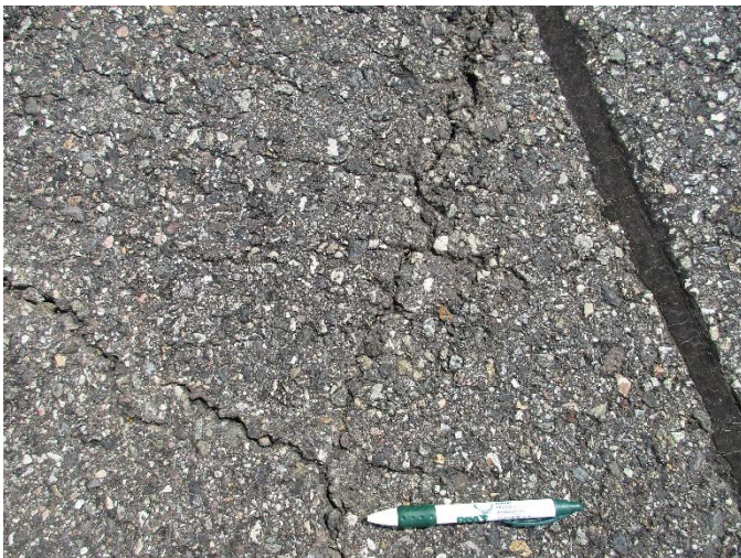
T-2, Surface detail with cracking & weathering
