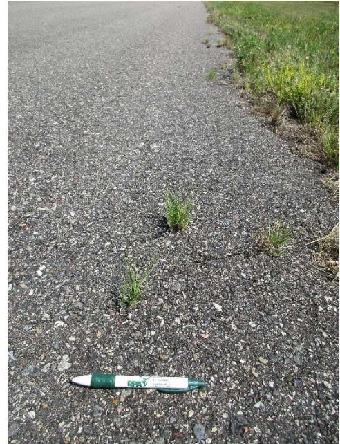
R-2, Surface detail with cracking & raveling (plant growth)
