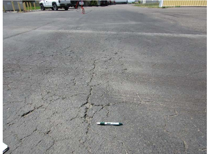
T-3, Surface detail with alligator cracking
