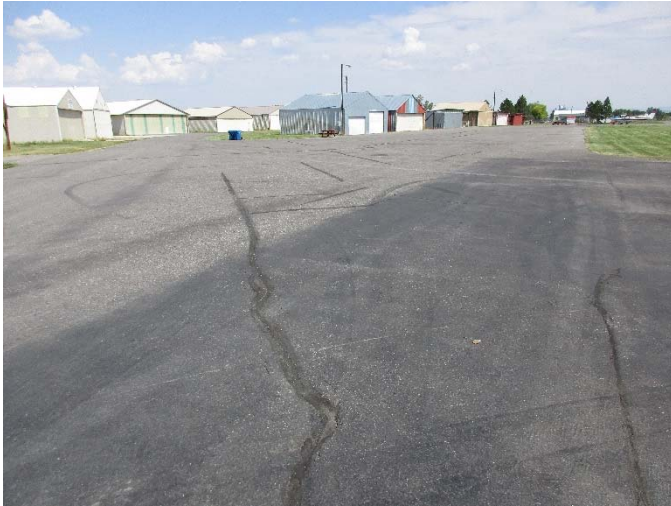
T-3, Overview with cracks
