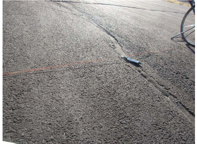
R-2 , Surface detail with crack & swell
