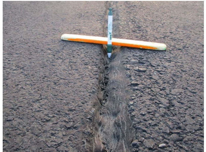
A-2, Surface detail with crack & depression
