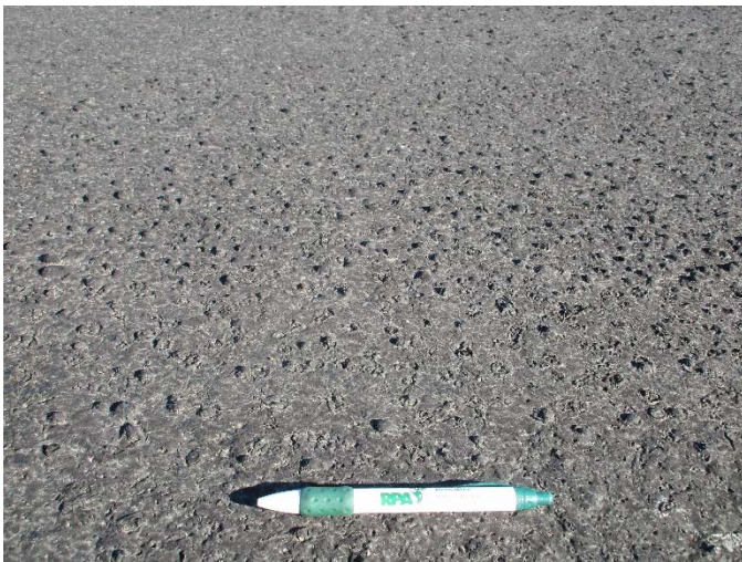
R-1, Surface detail with bleeding
