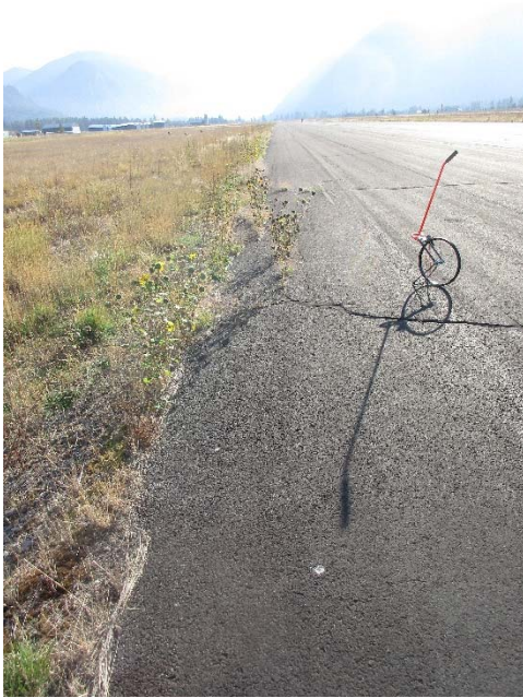
R-2 , Overview with weeds growing from cracks
