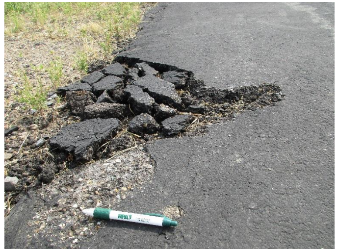
A-11 , Surface detail of severe mechanical damage
