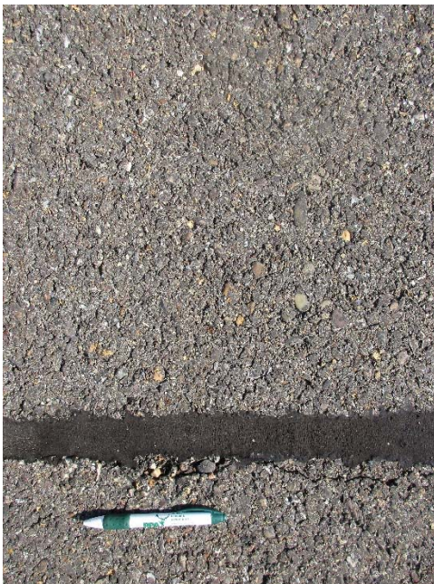
T-4, Surface detail with cracking
