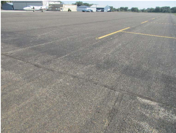
A-13 , Overview with scrapes / raveling
