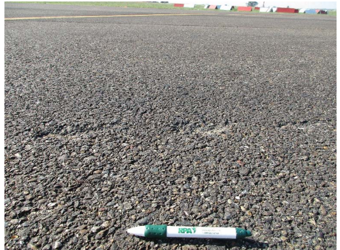
A-13 , Surface detail with gouges / raveling
