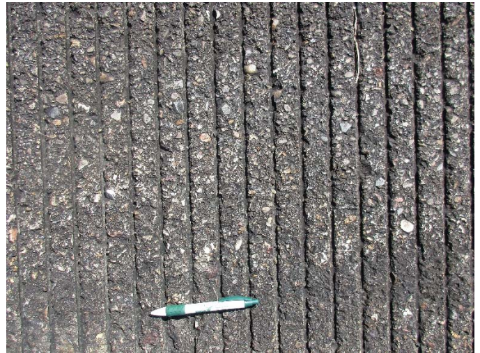
R-12, Surface detail with weathering & raveling
