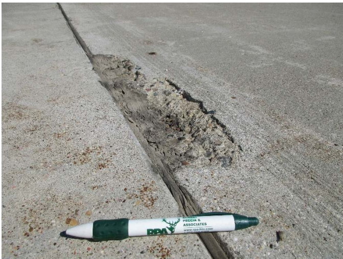
A-11, Surface detail with joint spalling
