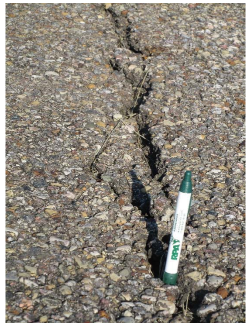
T-21, Surface detail with cracking
