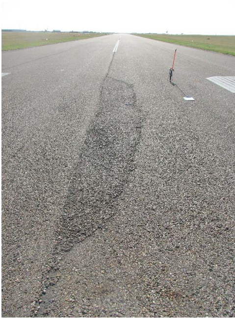
R-22, Overview with patching
