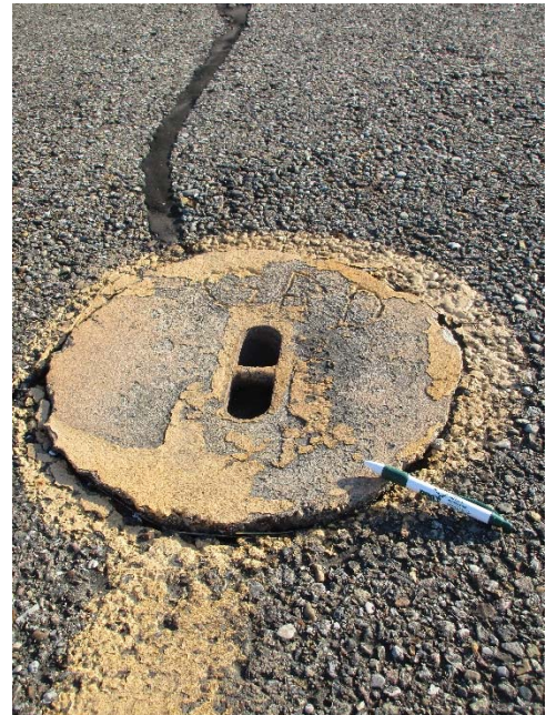
A-21, Surface detail with patch & swell
