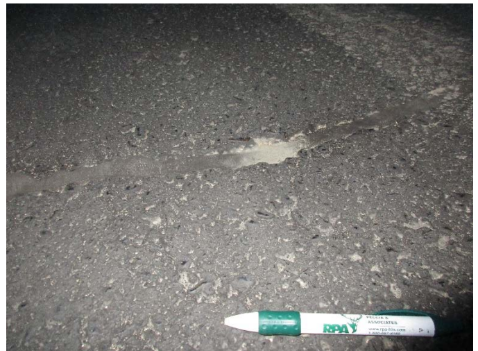
T-11 , Surface detail with cracking
