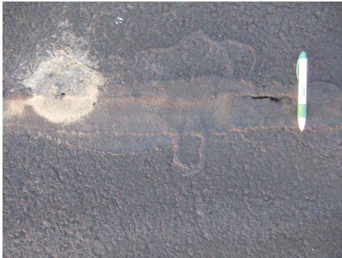
R-12 , Surface detail with partially sealed crack
