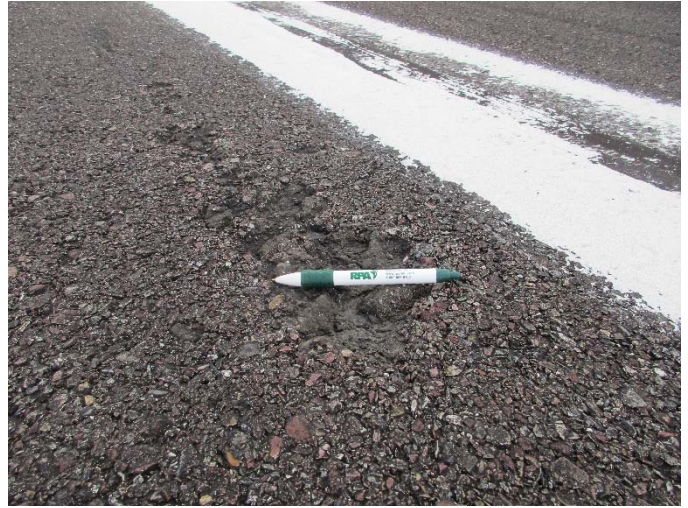
R-11, Surface detail with gouging / raveling
