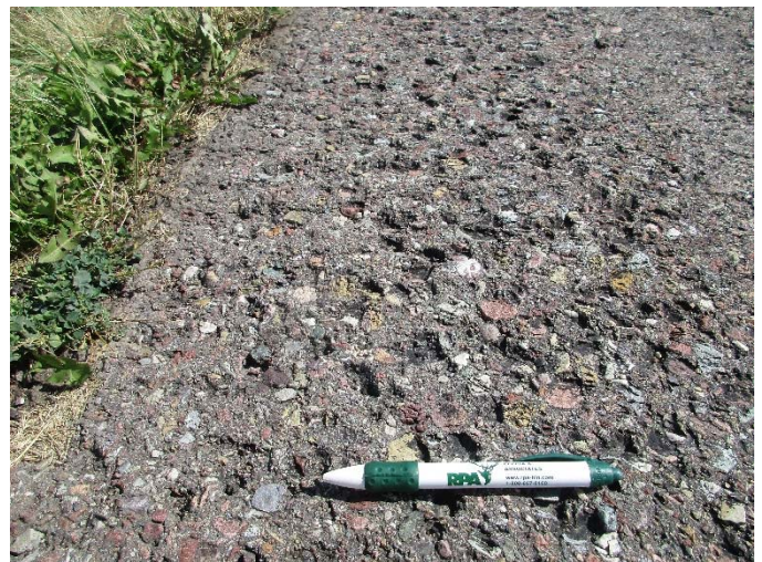
T-12, Surface detail with high raveling
