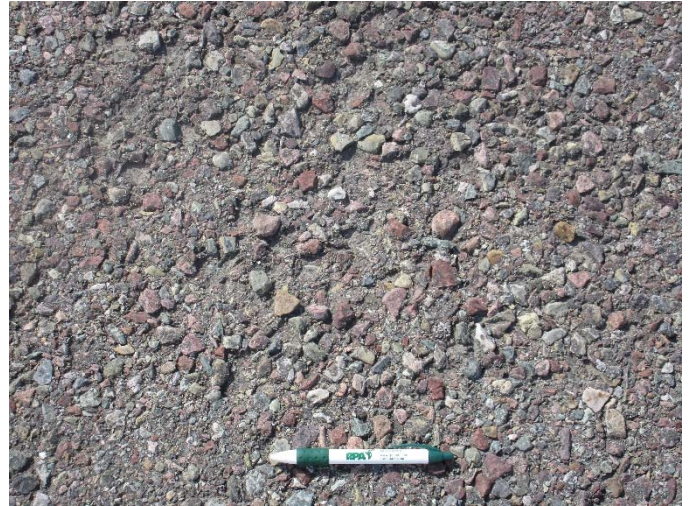
T-11, Surface detail with raveling
