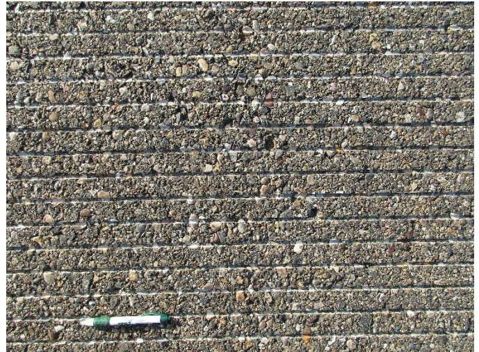
R-12 , Surface detail with grooves
