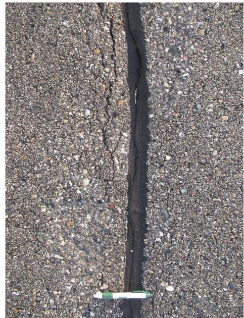
T-6, Surface detail with cracking
