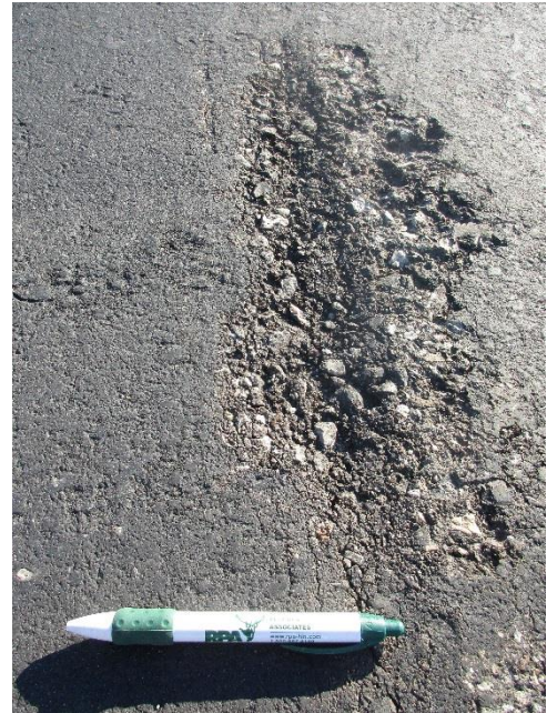
A-11, Surface detail with gouging
