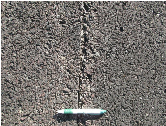
R-11 , Surface detail with cracking
