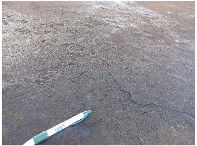
A-11, Surface detail with oil spill
