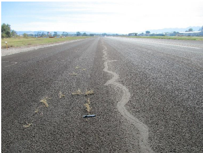
R-1A , Overview with grass growth from cracks
