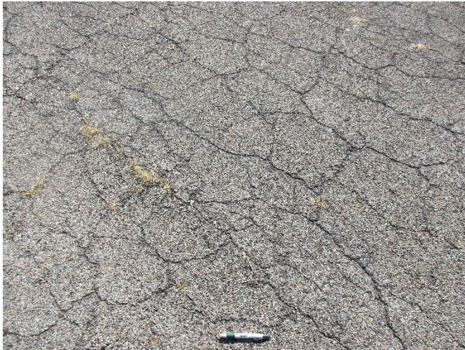
A-2 , Surface detail with alligator cracking
