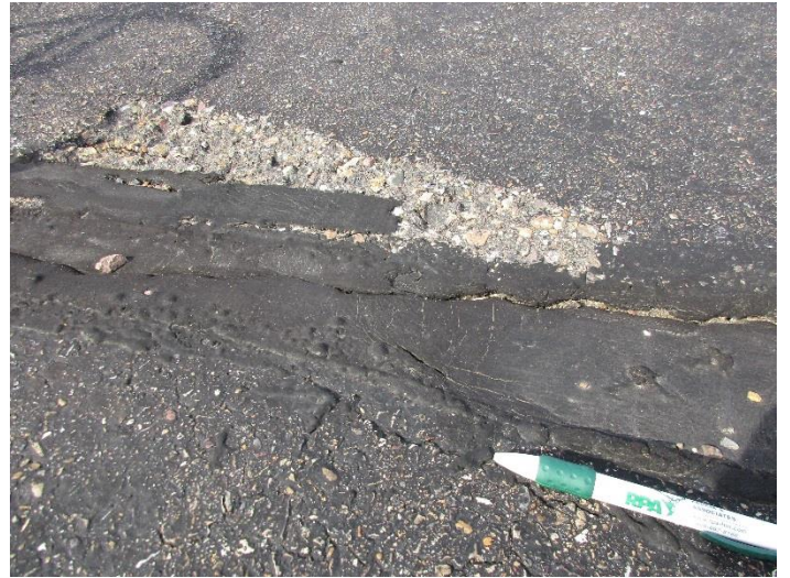
T-5, Surface detail with raveling and cracking
