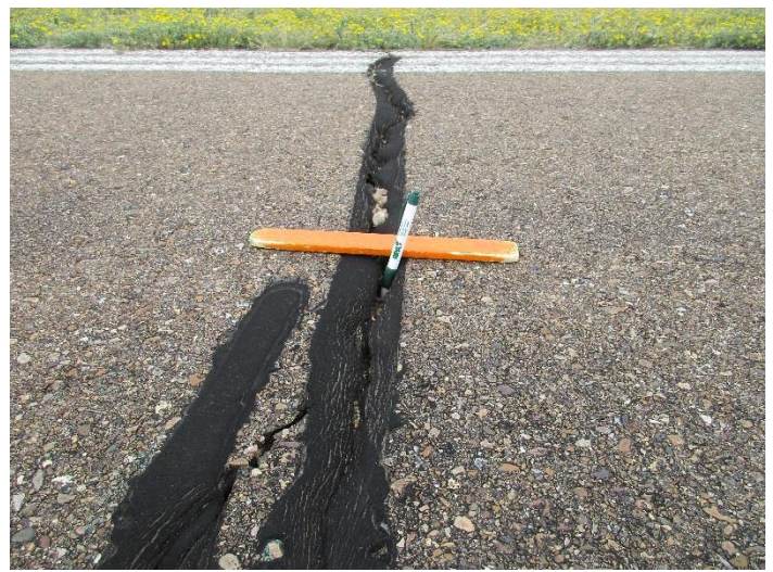
R-14, Surface detail with cracking
