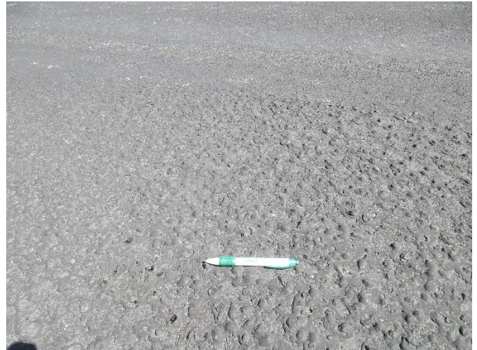
R-4, Surface detail with bleeding
