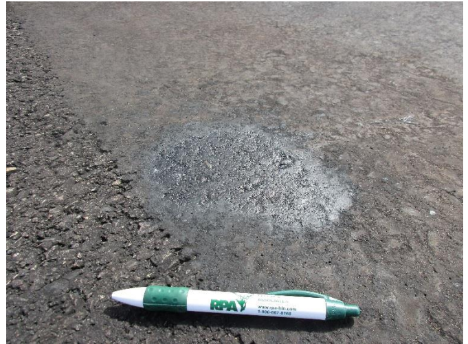
A-3, Surface detail with oil spill
