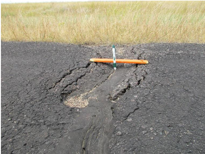
T-3, Surface detail with cracking
