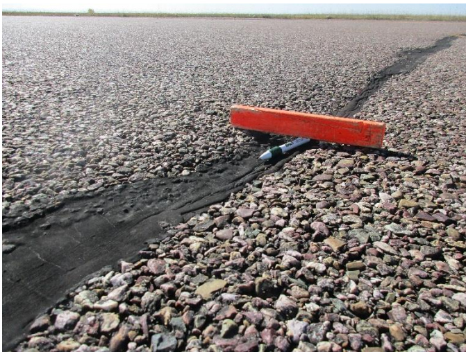
T-4, Surface detail with cracking
