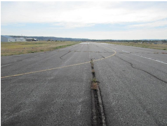
R-1 , Overview with cracking
