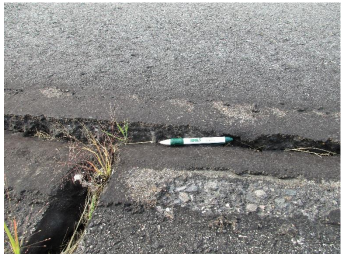
R-1 , Surface detail with cracking
