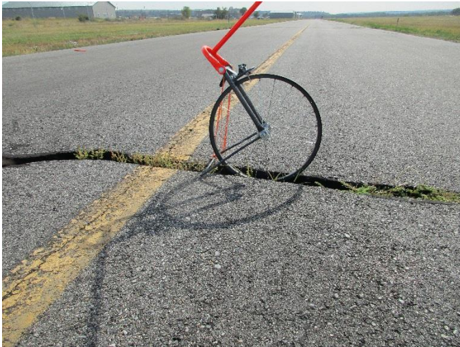
T-3 , Surface detail with cracking
