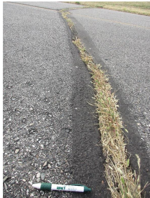
T-1 , Surface detail with cracking
