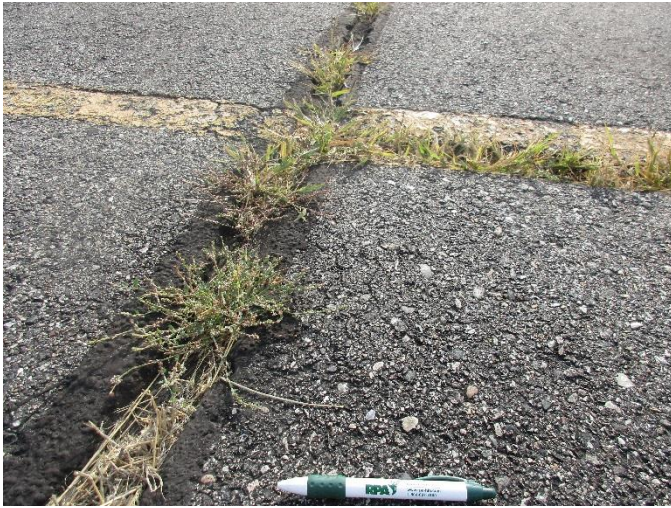
A-1 , Surface detail with cracking
