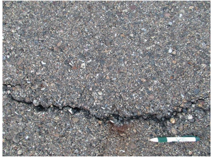
R-11 , Surface detail with cracking
