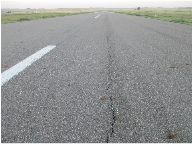
R-11 , Overview with cracking
