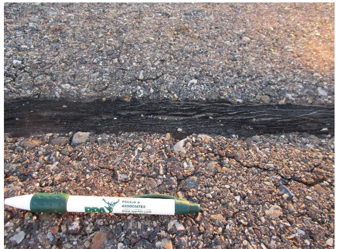
T-1, Surface detail with cracking
