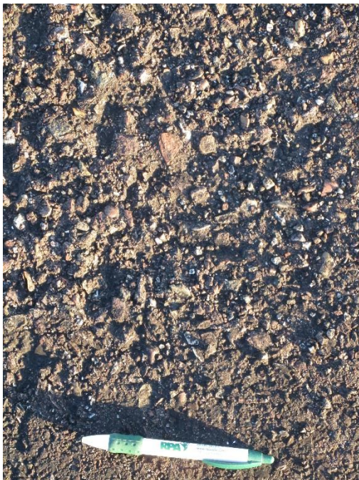
R-2 , Surface detail with raveling
