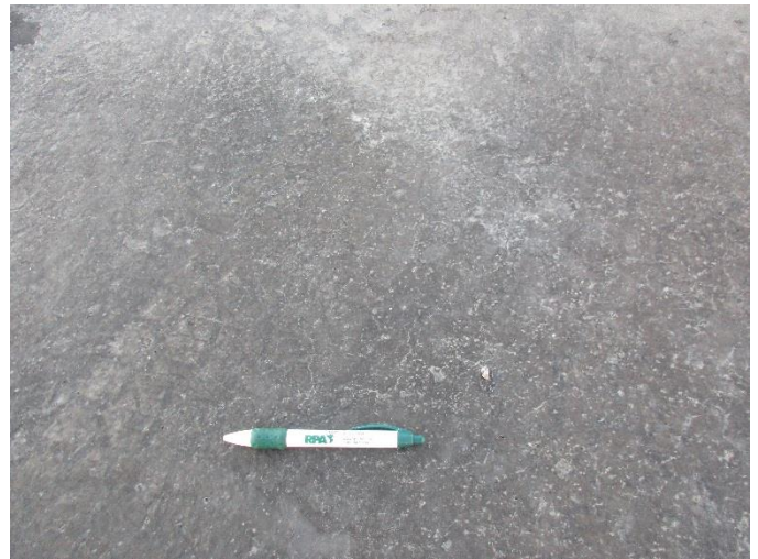
A-1 , Surface detail with bleeding
