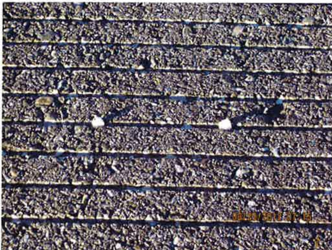
R-1, Surface detail with raveling
