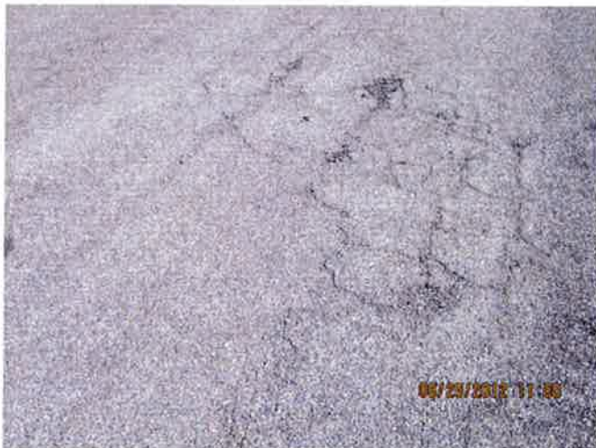
A-1, Surface detail with cracking
