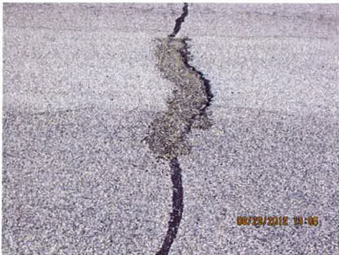
T-1, Surface detail with patch and crack
