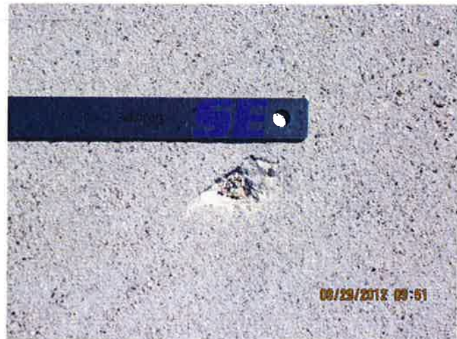
A-5, Surface detail with scaling
