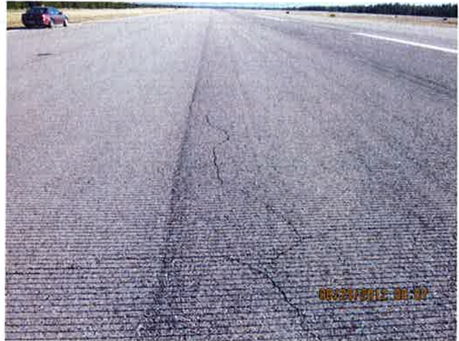
R-1, Surface detail with cracking
