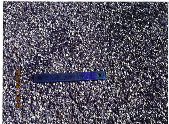
A-1, Surface detail with raveling
