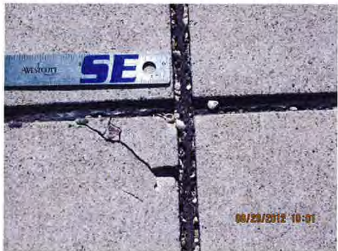
A-5, Surface detail with corner spalling
