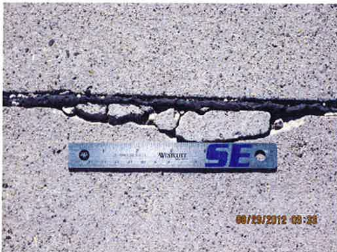
A-5, Surface detail with spalling
