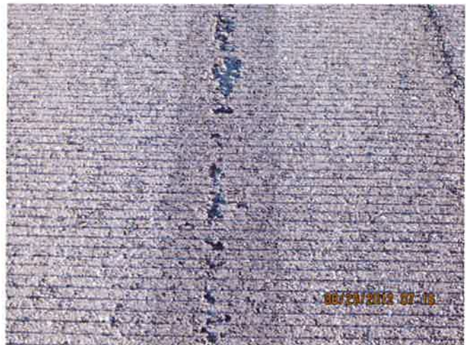
R-1, Surface detail with raveling 2
