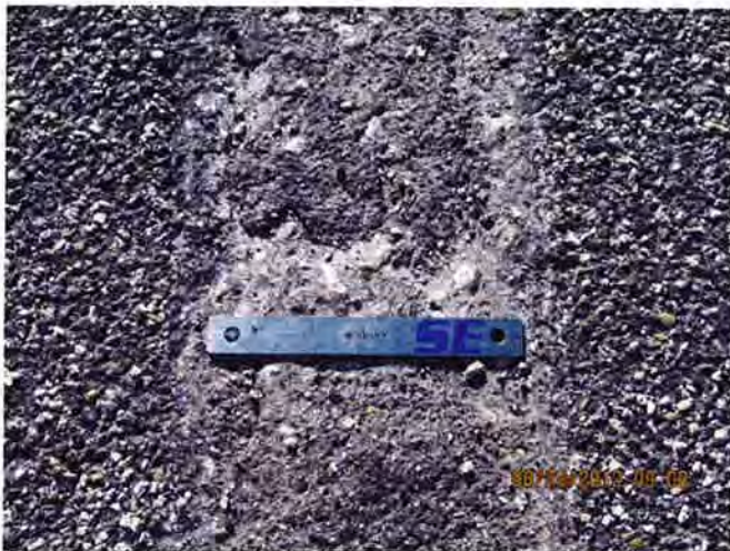
A-3, Surface detail with raveling
