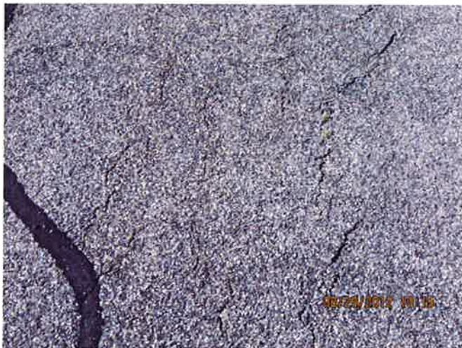
A-2, Surface detail with cracking
