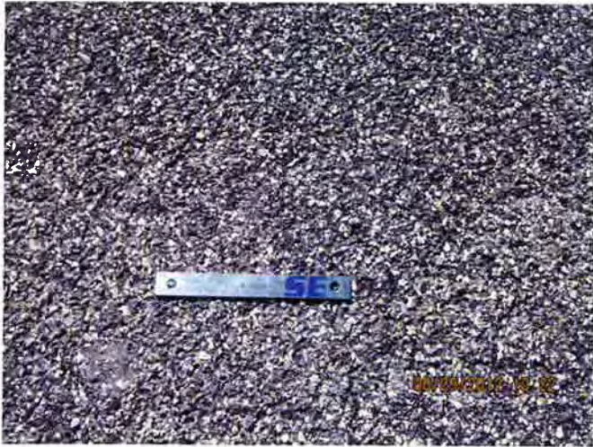
A-2, Surface detail with raveling
