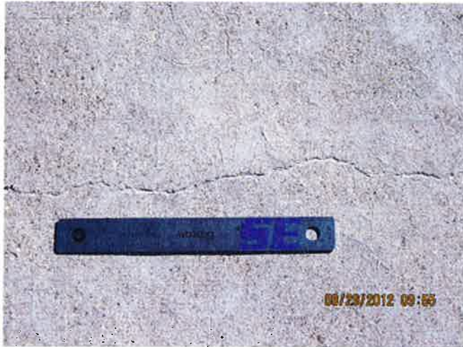
A-5, Surface detail with crack
