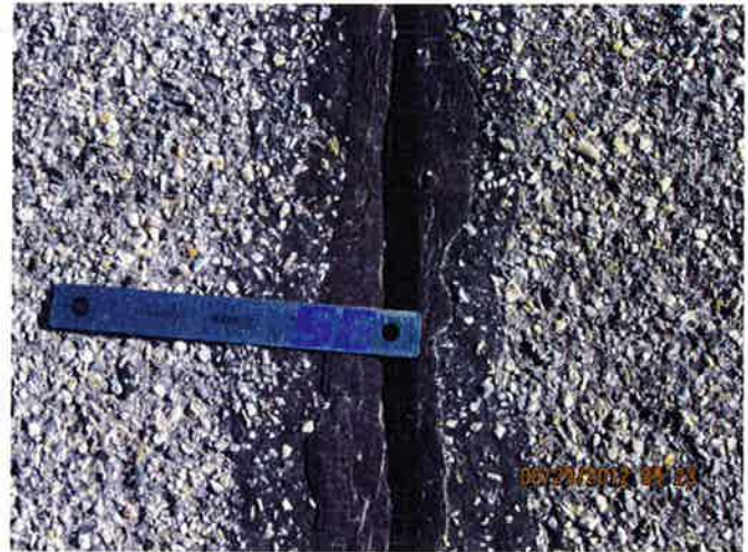
A-1, Surface detail with crack
