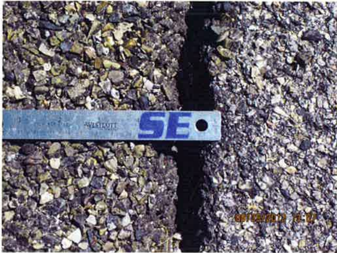
T-1, Surface detail with crack
