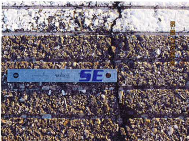
R-2, Surface detail with crack
