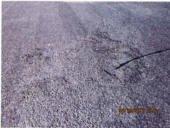
A-1, Surface detail with raveling 2
