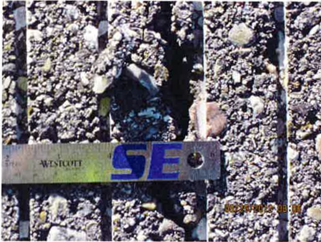
R-1, Surface detail with crack 2
