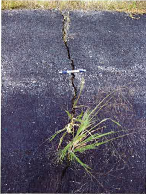
T-4 , Surface detail with crack
