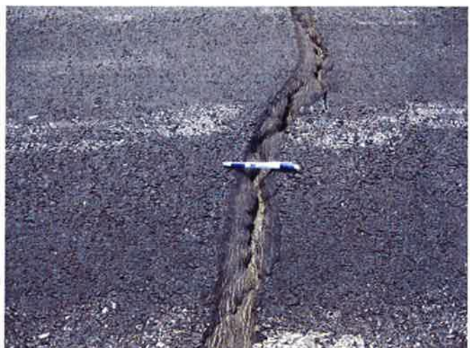
R-1, Surface detail with crack
