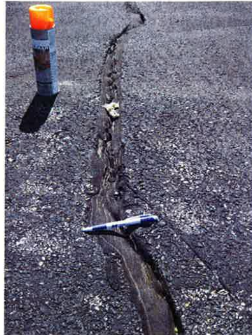
T-5 , Surface detail with crack
