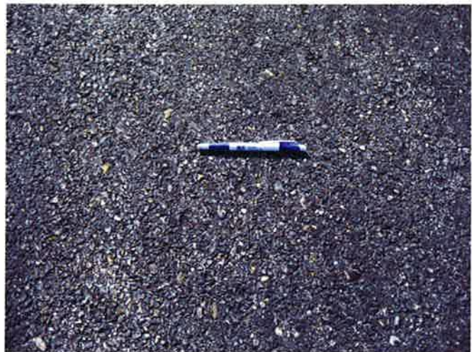
A-2, Surface detail with weathering
